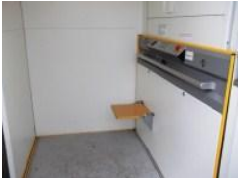
Example interior of access lift
