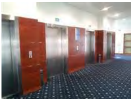
Lifts in ground floor foyer of the Millennium Grandstand leading to all floors
